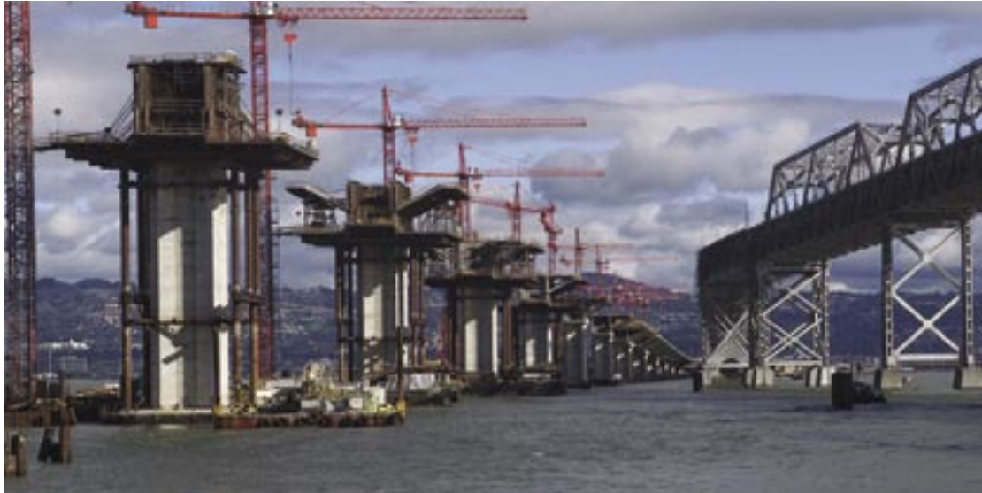
Figure 2. Construction of a replacement bridge for the East Bay is proceeding parallel to the original span, which remains open to traffic. (Photograph courtesy of John Huseby/Caltrans.)
